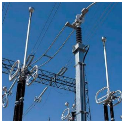
High voltage bushing
