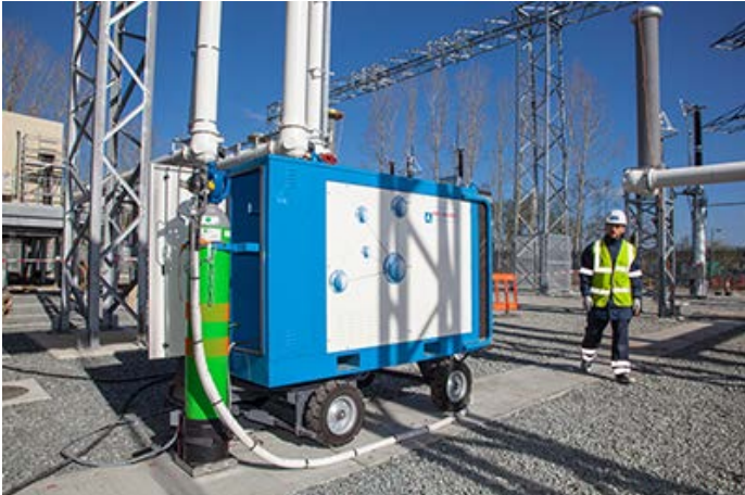
Figure 4: Air Liquide's g 3 -filling cart in service at a National Grid site in the UK
