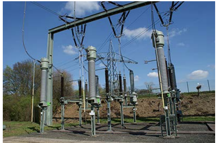
Figure 3: An SF_6 -free 245 kV current transformer using g^3 installed at a TenneT substation in Germany
