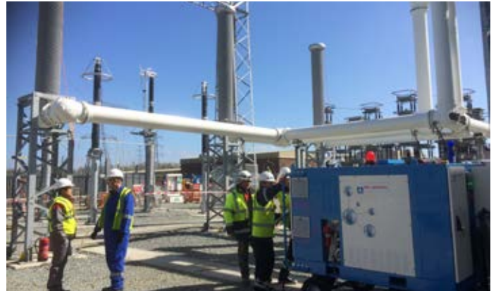
Figure 10: g 3 -filling of the 420 kV GIL at National Grid's Sellindge substation, UK
