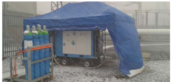
Figure 11: g 3 -filling under harsh weather conditions of the 420 kV GIL for Scottish Power's Kilmarnock substation, UK
