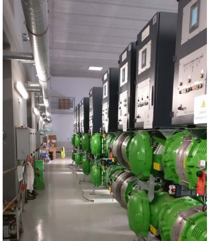
Figure 15: 72.5 kV F35 GIS using g^3 installed in RTE's Grimaud substation in France
