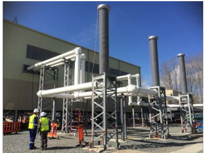
Figure 2: A 420 kV gas-insulated line filled with g^3 at National Grid's new Sellinglee substation in the UK
