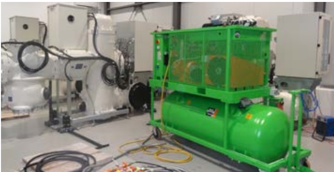
Figure 13: DILO's g^3 -service cart used at Axpo's Etzel substation
